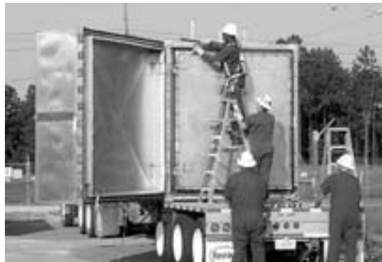
Savannah River Site riggers Lawrence Smith, Ken Wood, Bobby Lowe, and Benjamin McClain open the internal door of the TRUPACT-I before shipment. The door has 26 bolts that must be removed before the door can be opened.
