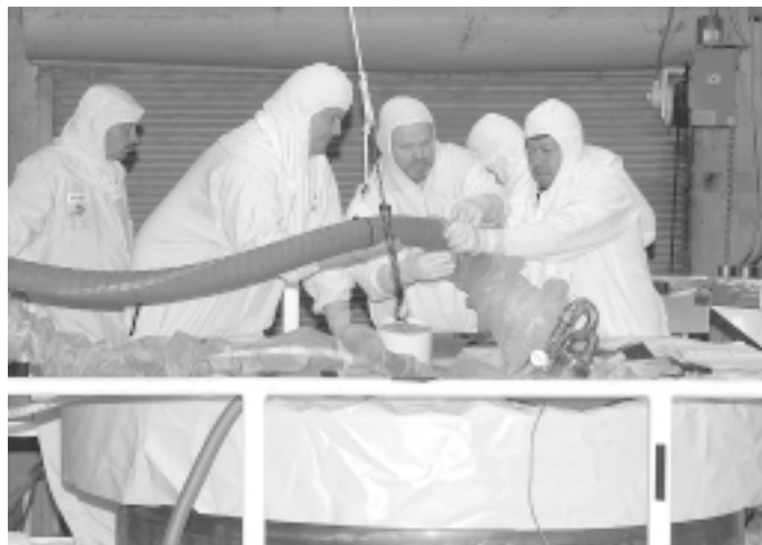
Workers connect hoses to ports in the top of Large Diameter Containers that will hold sludge from the North Loadout Pit in the K East Basin until it can be grouted later this year.
