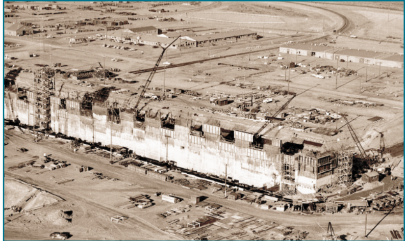
Figure 8. PUREX Plant, shown under construction in 1954, produced about 50% of the U.S.-produced recycled uranium.
