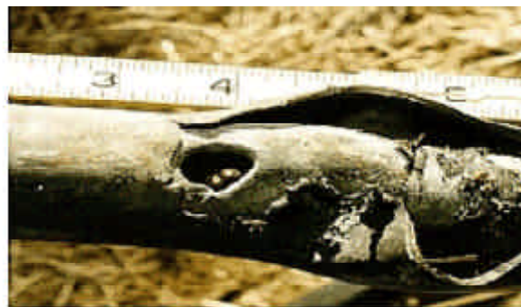
Figure 3. Penetrated 13,200-volt cable during construction
