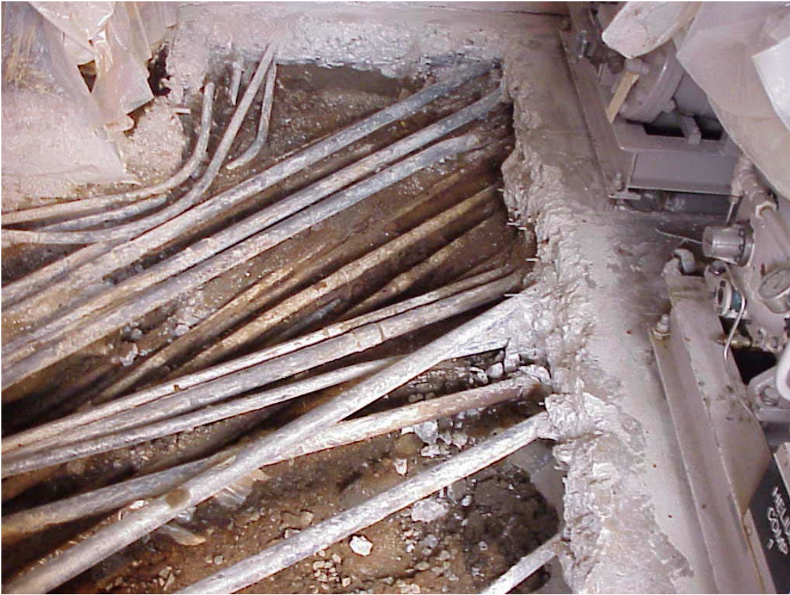
Figure 1 – Conduit exposed during concrete removal to perform soil sampling. This illustrates the challenges in avoiding electrical conduit during surface penetration activities.
