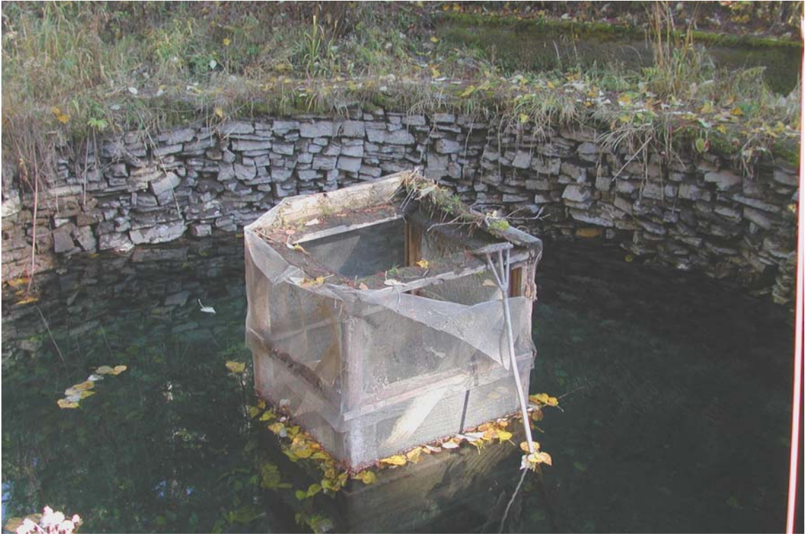
Figure 48. City of Troy water cistern O'Brien Creek, with old outlet pipe screen cover.
