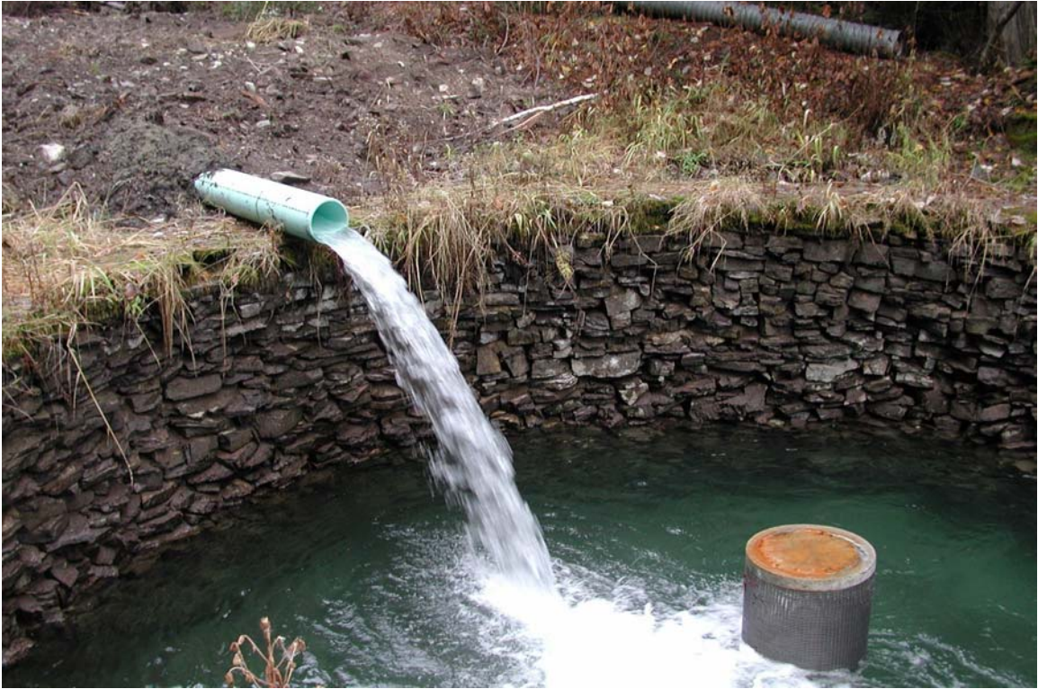
Figure 49. Troy water cistern O'Brien Creek, after change in diversion and installation of new outlet pipe screen cover.
