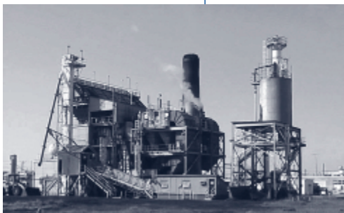
The boiler plant at the Department of Energy's Savannah River Site cofires coal and biomass.
