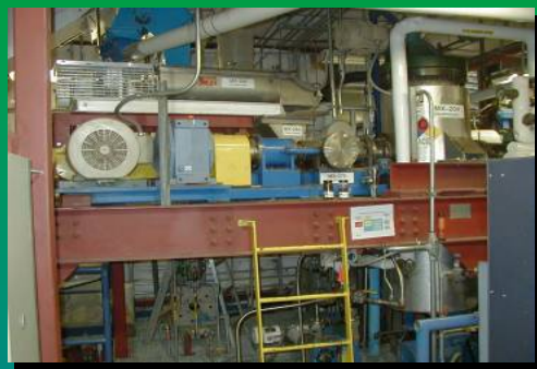
Sands vertical reactor for pretreatment of corn stover.
