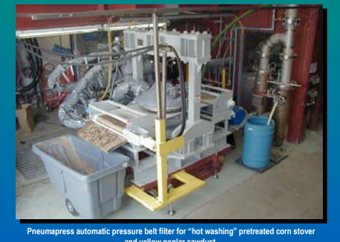
Pneumapress automatic pressure belt filter for "hot washing" pretreated corn stover and yellow poplar sawdust.
