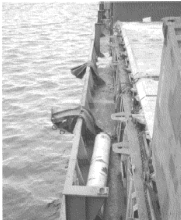
Failed deck pedestals (starboard side locking aft)
