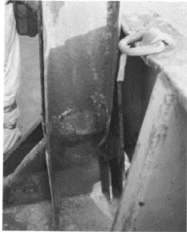
Compression damage at bottom of pedestal
