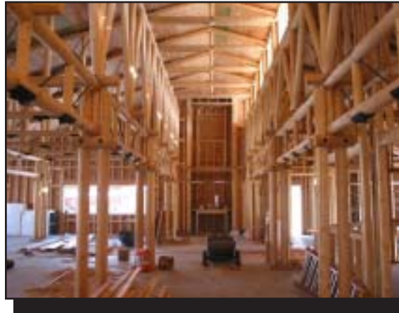
Small, roundwood trusses throughout the main room of the public library in Darby, MT.
