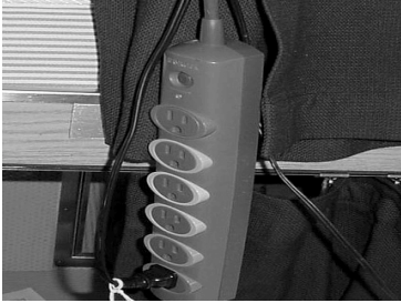
Unapproved Power Strip
