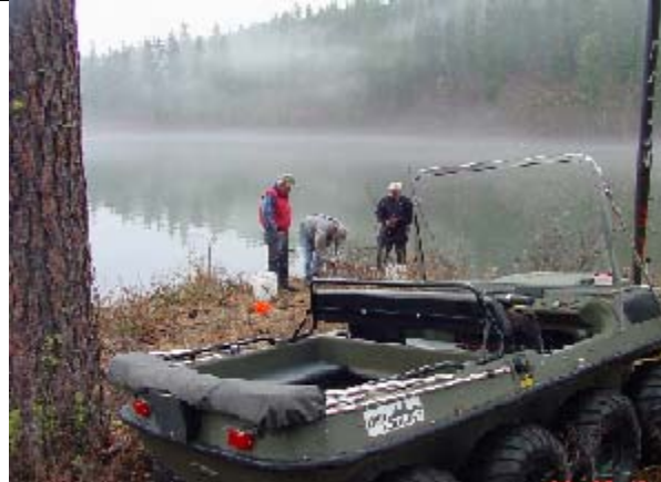
Photo 1. South facing view of Little Owhi Lake located approximately 1.5 miles north of Big Owhi Lake on the Colville Confederated Tribes Reservation, WA. Photo also depicts fishery technicians installing solar power aeration system supports.
