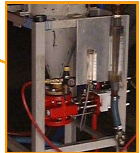
Control instruments and discharge valve mounted on the CrossFlow unit.
