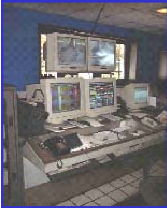
Computer-based interface used to monitor and control the heavy media bath and heavy media cyclone circuits at one of the four project test sites.
