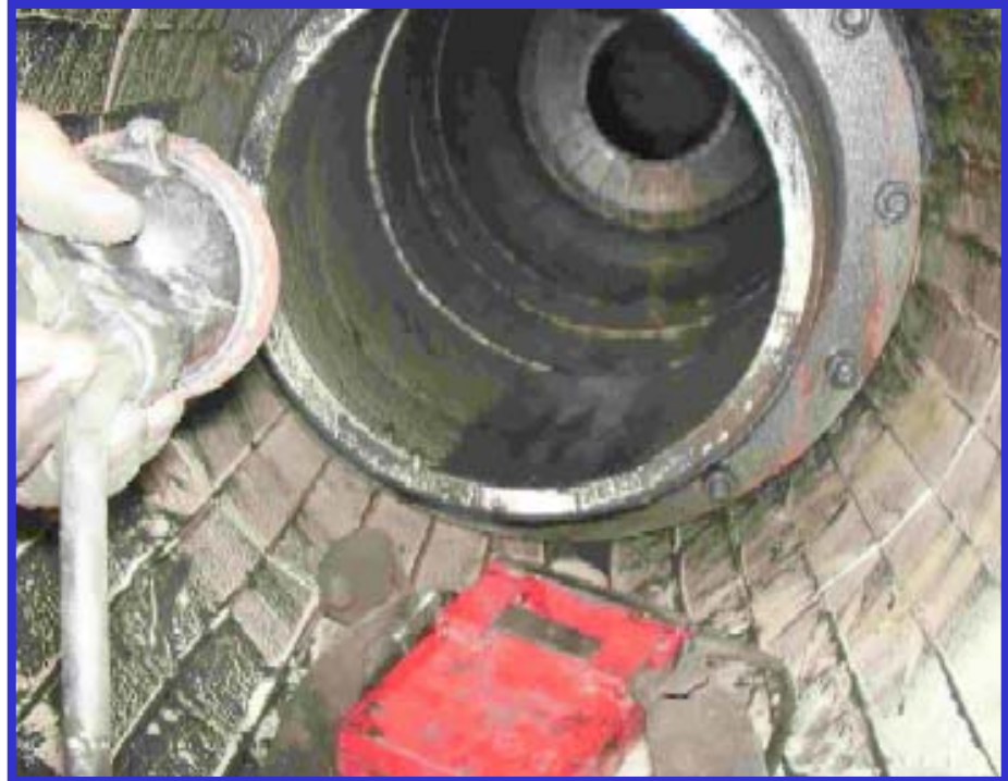
Photograph showing the internal condition of one of the heavy media cyclones (ceramic lined) that was inspected by the project team during the first phase of the in-plant test program.
