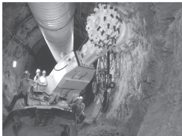
An "alpine miner" excavates an access tunnel inside Yucca Mountain. The Office of Civilian Radioactive Waste Management continues to conduct site characterization studies of the Yucca Mountain Site.
