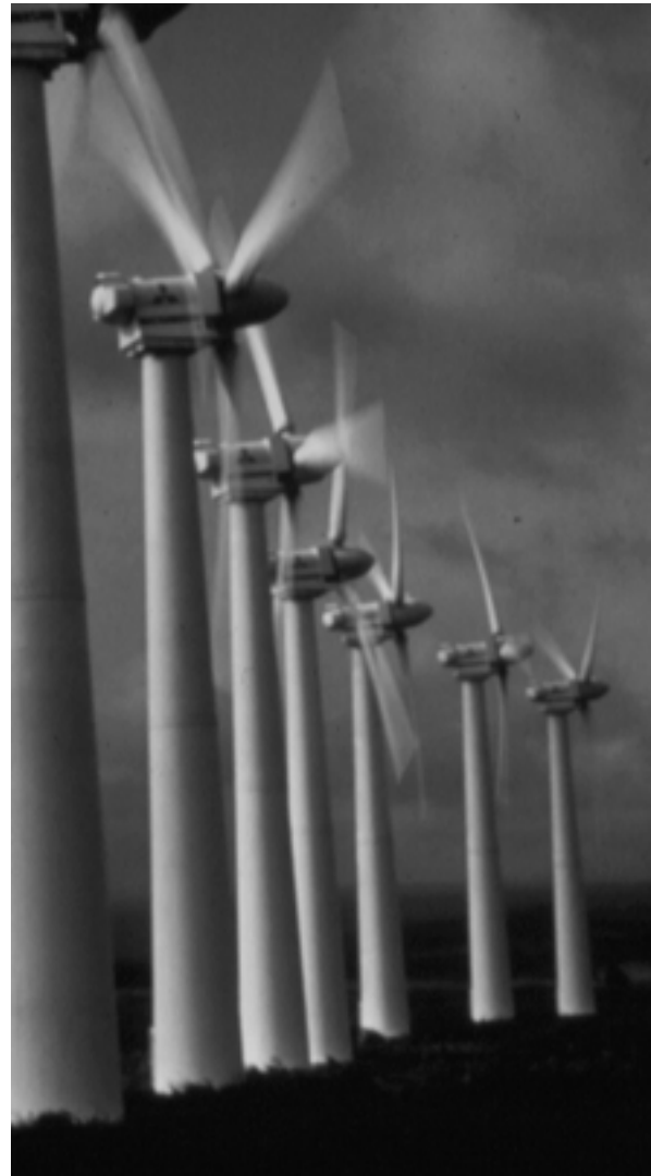
Figure 3. Tubular towers in a linear array in South Point, Hawaii. Photo by Paul Gipe.
