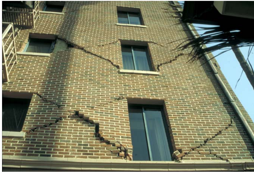
Figure 2.6 Structural damage to masonry building resulting from the 1994 Northridge, California, earthquake. Reproduced courtesy of the National Information Service for Earthquake Engineering, University of California, Berkeley.
