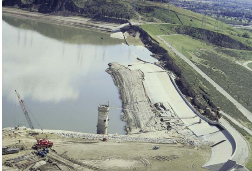
Figure 2.4 Embankment failure due to liquefaction at the Lower Van Norman Dam, 1971 San Fernando, California, earthquake. Reproduced courtesy of the National Information Service for Earthquake Engineering, University of California, Berkeley.
