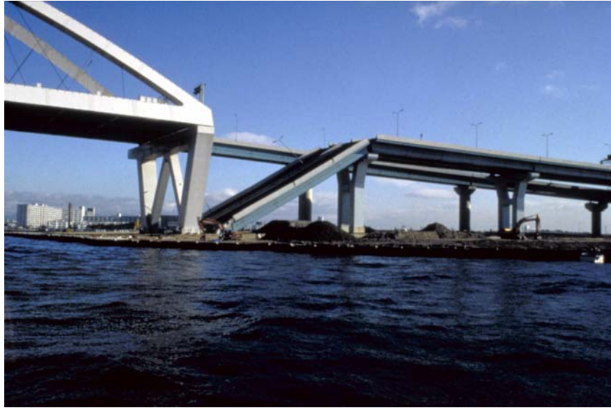
Figure 2.8 Failure of a span of the Nishinomiya Bridge during the 1995 Kobe, Japan, earthquake. Reproduced courtesy of the National Information Service for Earthquake Engineering, University of California, Berkeley.
