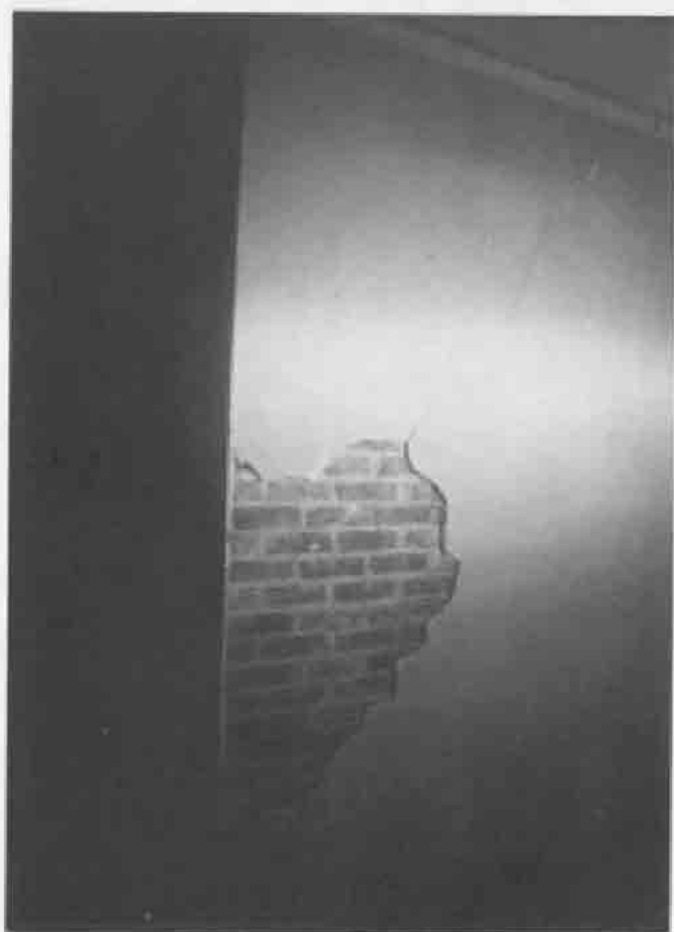
Alice's Room: Plaster Damage
