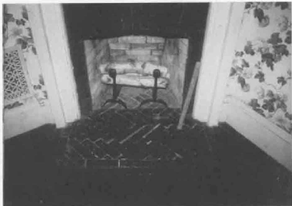
Mother's Room: Condition of Fireplace Hearth Before Restoration
