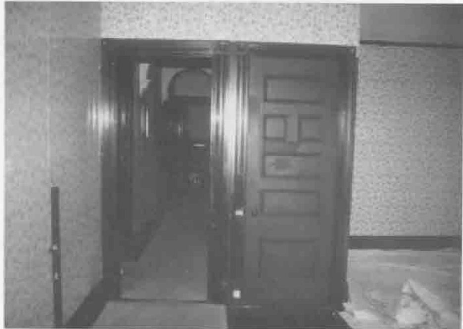
Typical Condition of Stained Woodwork
