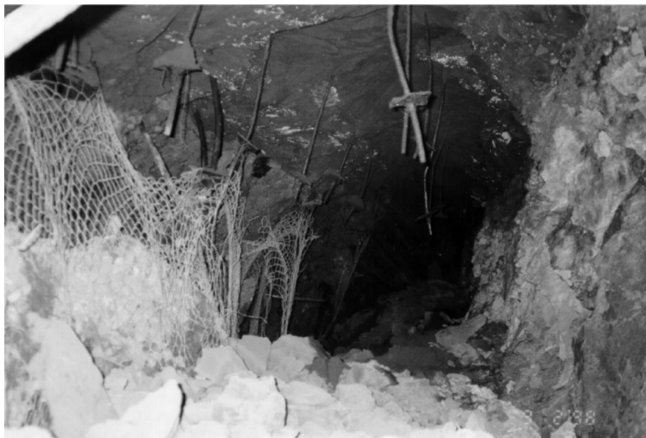
Figure 2. Rock burst damage in the 5750-05 stope. Note that both ribs, as well as the overhead sandfill, were damaged in this event.
