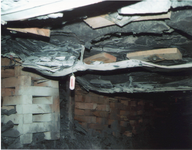
Figure 16. Rear abutment stress damage in the L1 entry
