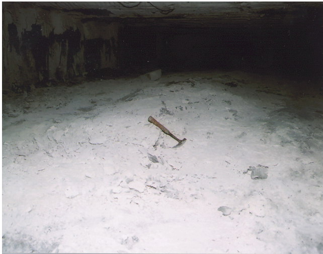
Figure 12. Floor heave experienced in E15 panel.
