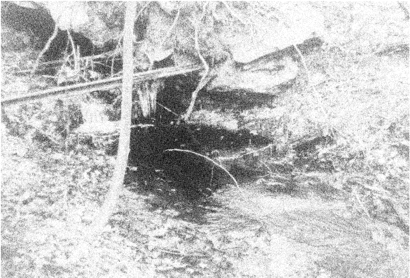
Example of abandoned underground mine exhibiting exposed mine entry and mine drainage
