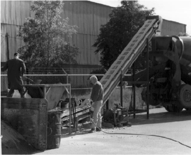
Conveyor system used to load dry total tailings into ready-mix truck.
