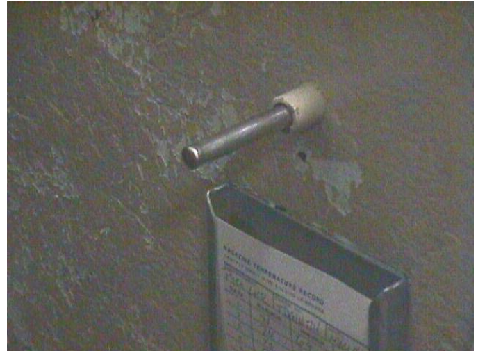
View of incorrect/altered thermometer well
