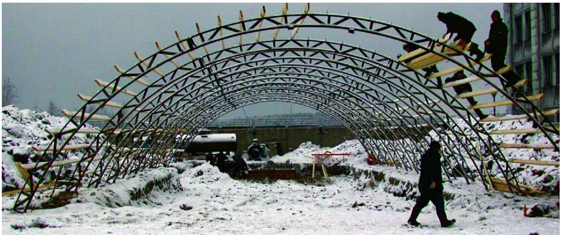
TOBOS, the Russian acronym for Safety and Security Technologies for Russian Warheads, included construction of all-weather enclosure that allowed crews to repeatedly heat and remove 1.5 meters of permafrost each day in order to pour the foundation of the TOBOS test facility.
