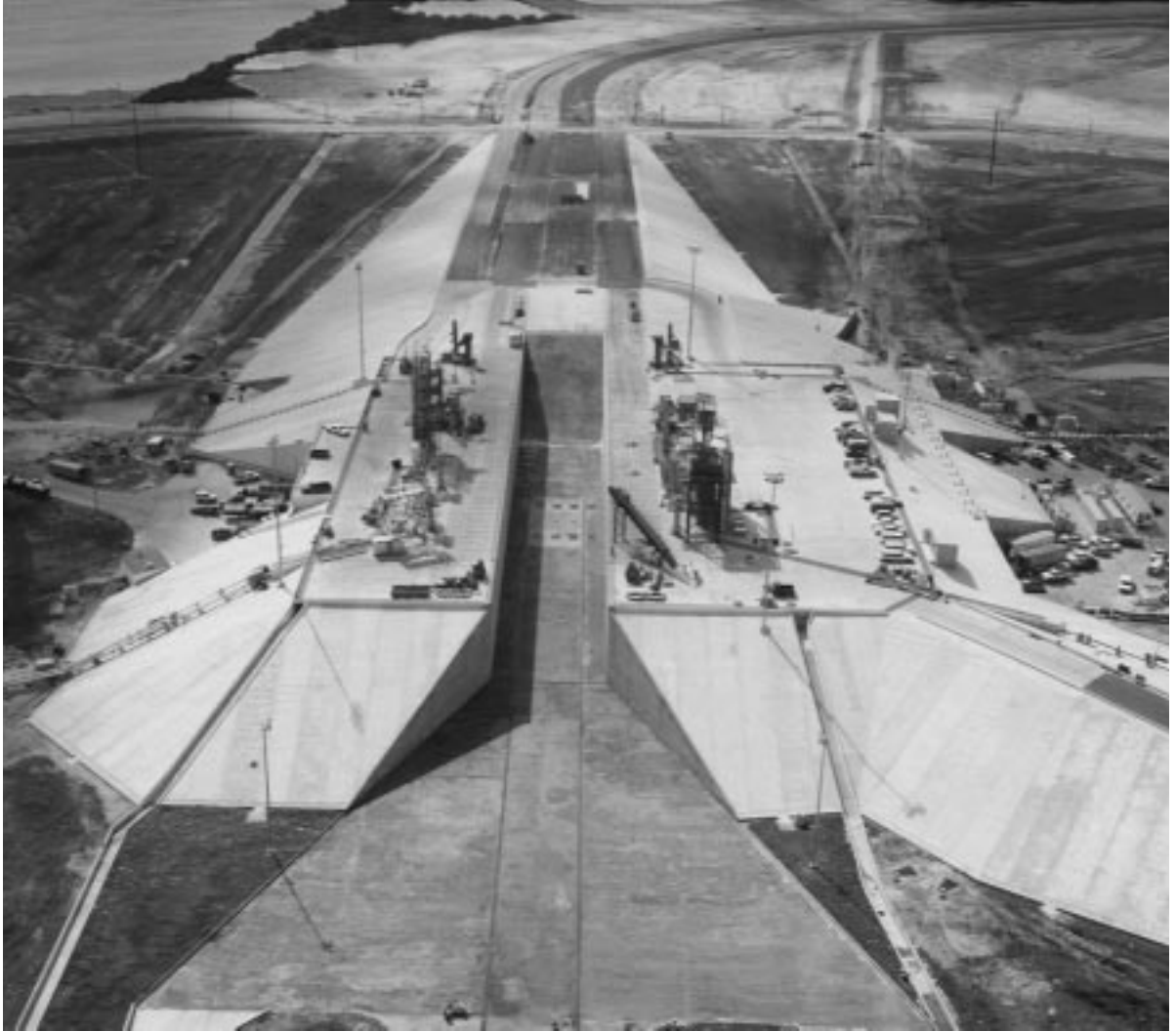
Construction of Pad A at Spaceport's Launch Complex 39. The pad hardstand contains 68,000 cubic yards of concrete.
