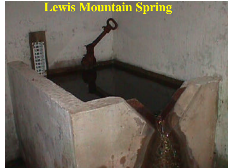
Sampling from a Typical Spring Box and Weir
