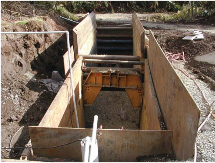
FIGURE. This properly installed support system for trench work includes a shoring system with crossbracing and vertical plates extending at least 18 inches above the lip of the trench
