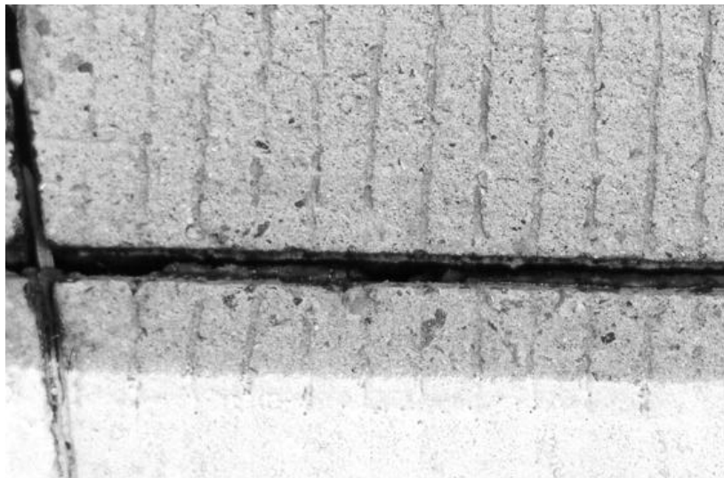
Figure 3. Full-depth cohesion failure.
