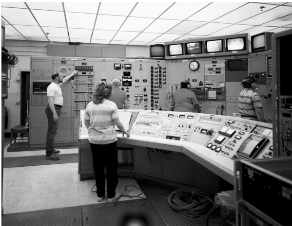
Control room of the 8-Foot High Temperature Tunnel.
