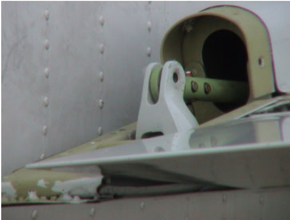
Figure 11. Photograph of the test airplane's disconnected right elevator control tab pushrod centered between the lugs of the crank fitting with the control tab rotated 3° to 4° in the TEU direction after the attachment bolt was removed.
