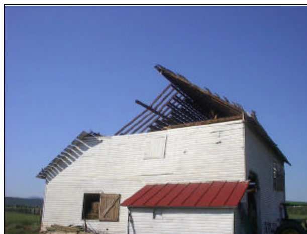
A F1 tornado damaged a barn in Madison County
