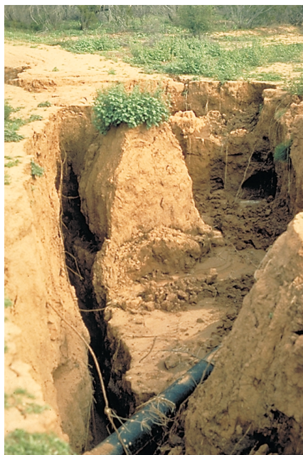
A natural-gas pipeline undercut by an earth fissure was exposed through erosional widening of the fissure. The pipeline was evacuated and cut to determine the stresses on it. Tension was evident, but no shear.
