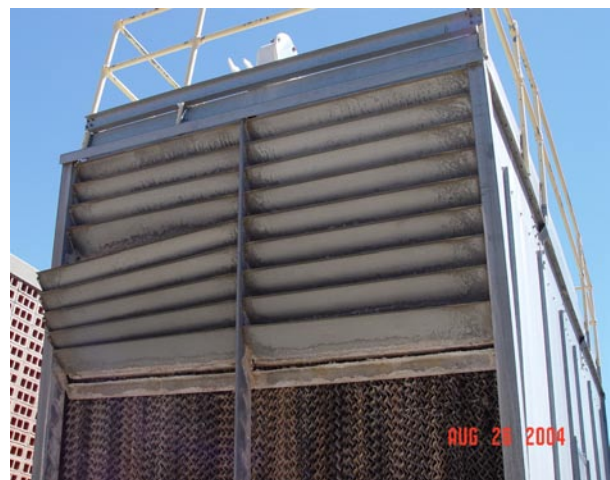
Figure 2-1. Cooling tower and fill material
