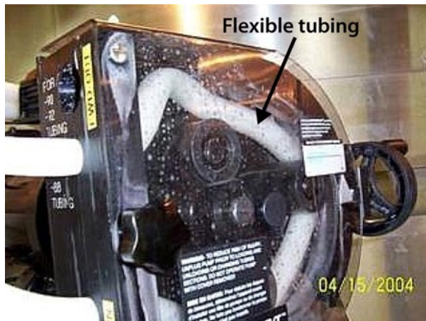
Figure 4-1. The pump shortly after the accident
