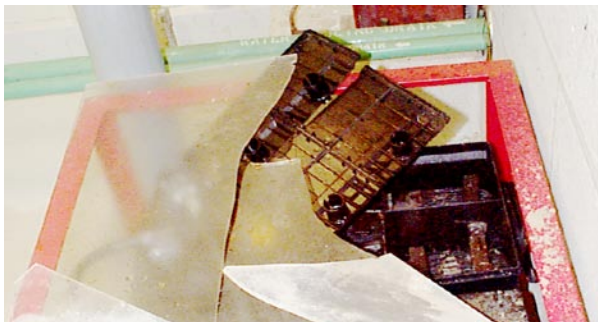
Figure 4-3. Damaged plastic cover over battery bank
