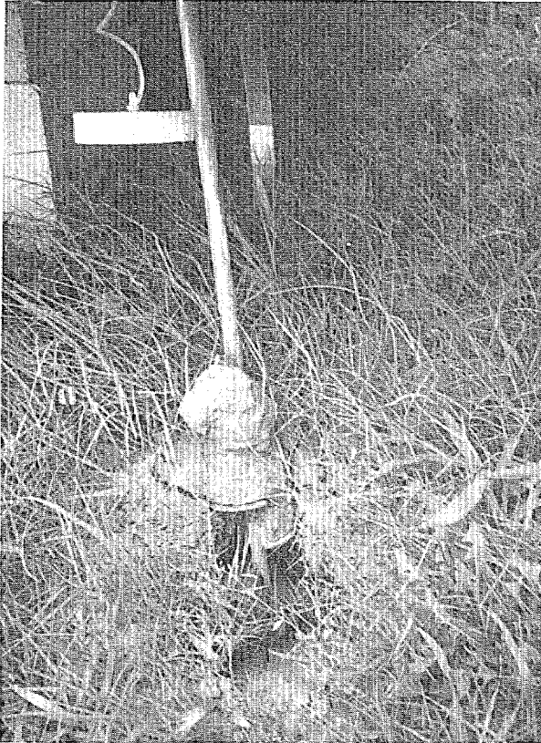
Figure 1.25 Failed Ground Anchor
