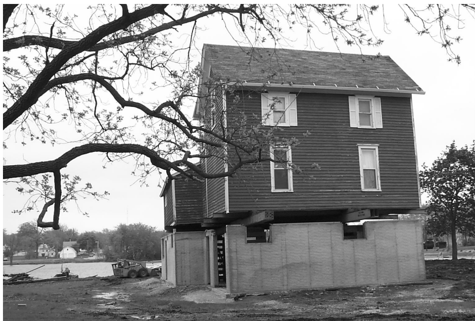
At first, said Joni Hocken, their Independence, Iowa, neighbors were puzzled by the spectacle of their 100-year-old, two-story, red-painted home being elevated on new concrete foundation walls. (Photo: Mike McCoy, FEMA)
