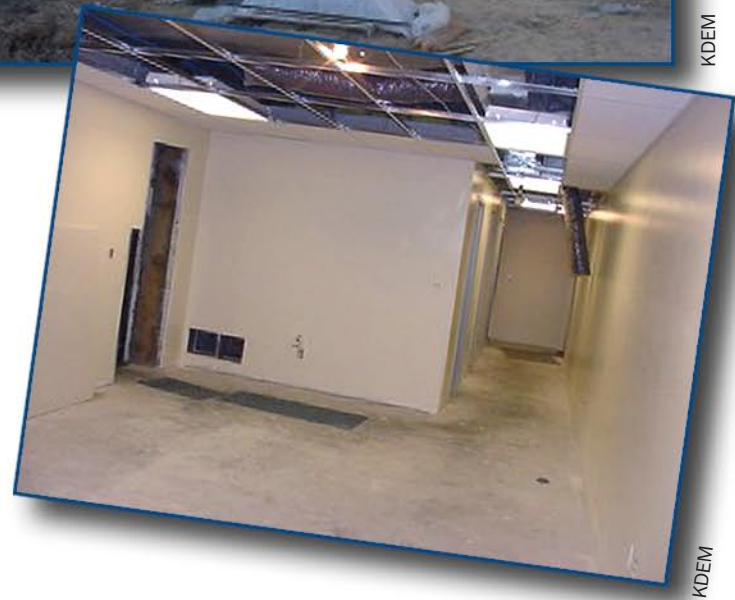
Construction of the reinforced ICF exterior wall at the rear of the shelter (top). Interior walls of shelter with gypsum board finish (bottom).
