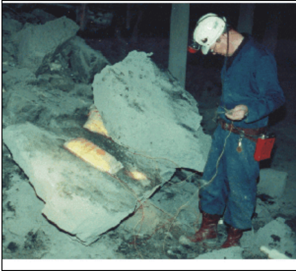
A Rock Buster is used to remove a roof fall.
