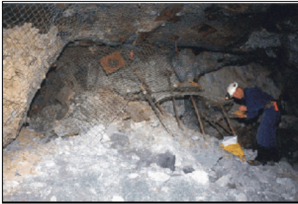
Rock burst damage in a hard-rock mine.
