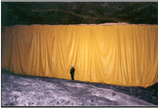
One of three brattice cloth ventilation stoppings installed in the Lake Lynn mine for this project.
