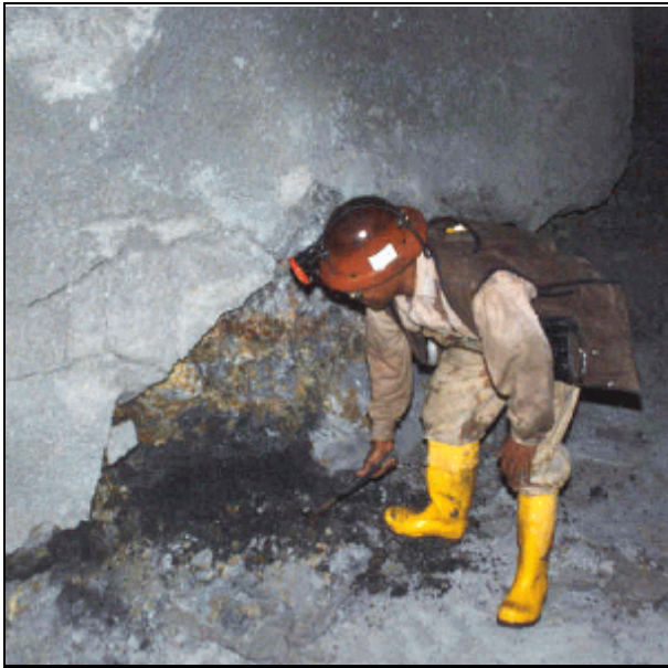
Rib failure at an underground gold mine in Nevada.
