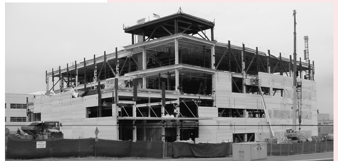
The NISC building, which is about 1/3 complete and $1M ahead of schedule.
