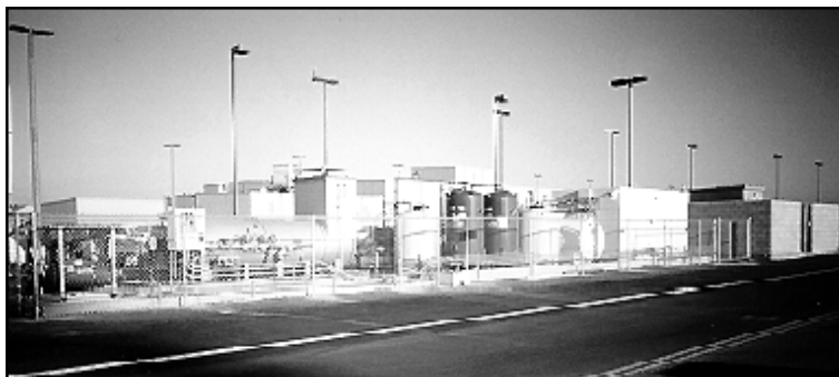
Figure 3. Functioning Extraction and Treatment System
