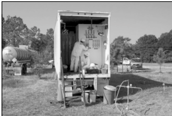
Chemical Oxidation Process Controls in Tractor Trailer and Hydrogen Peroxide in Tanker Truck (injection well, foreground)
