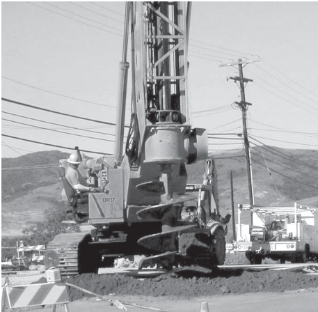
Figure 1. Large-diameter drilling rig with a 4ft. diameter auger at Camp Pendleton site.
