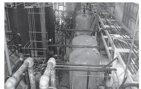
Figure 3. Interior of support building for closed loop steam heating remediation process.
