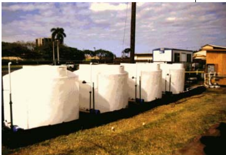
Figure 1. Storage tanks used for blending electrolyte solutions.
