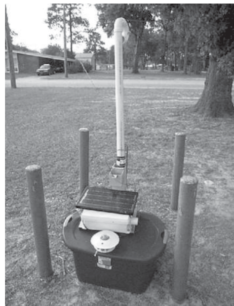
Figure 2. Example vent well equipped with monitoring equipment to collect performance data.
