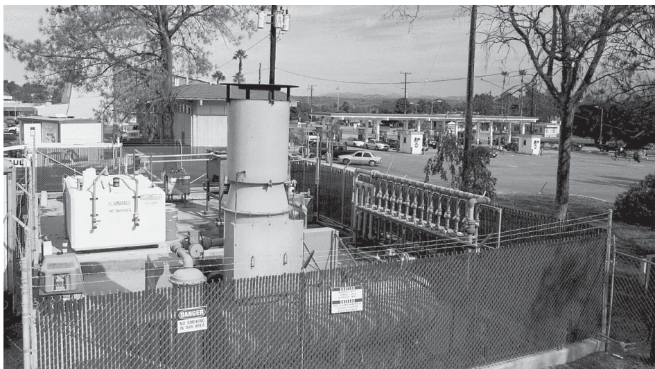
Figure 1. Overview picture showing treatment compound in foreground (including fluid storage system, vapor extraction manifold, and oxidizer) and gas station in background.
