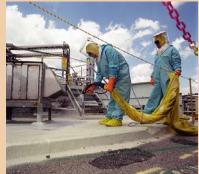
Savannah River Site workers apply Instacote to large equipment as an alternative to size-reduction
