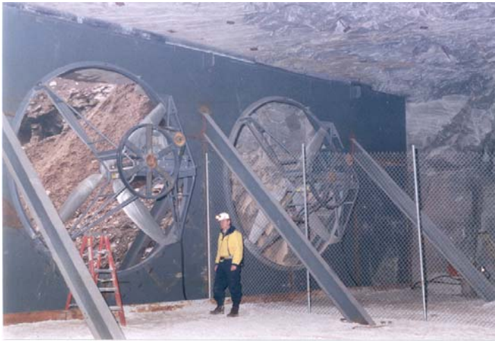
Figure 1.—Two propeller fans installed in an underground stone mine.
