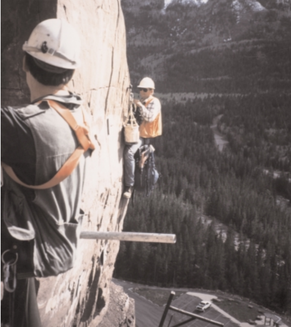
Where do Interior's scientists work? On the ice in Antarctica, inside the caldera at Mount St. Helens, or here, on a rock face 200 feet above Upper Stillwater Dam, where Bureau of Reclamation geologist Mark Neely installs monitoring equipment on potentially unstable rock.
