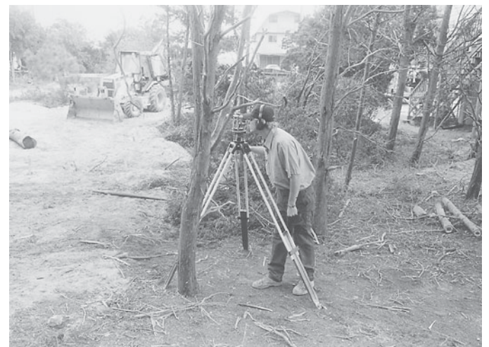
Surveyors select known survey reference points and determine the precise location of important features in the survey area.
