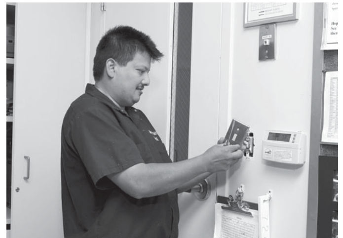
General maintenance and repair workers in small establishments, where they are often the only maintenance worker, do all repairs except for very large or difficult jobs.
