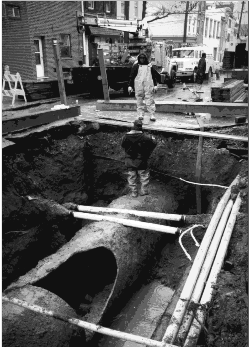
Figure 1: Decaying Drinking Water Pipeline in Philadelphia
